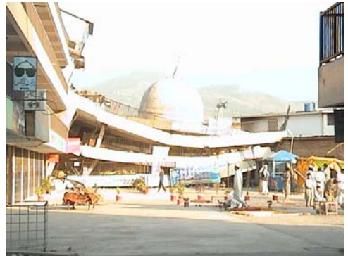
Abbotabad: Collapsed market in Abbotabad, photo by CESNED team
