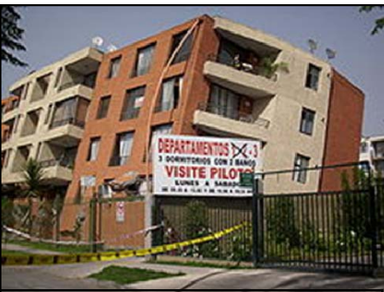
Fig 10: A severely damaged building in Maipú, Santiago
