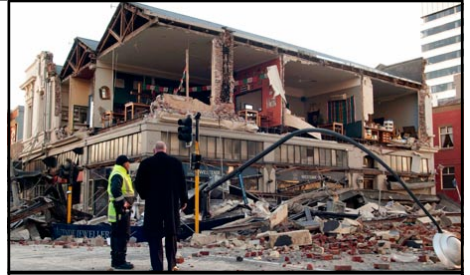
Fig 9: Earthquake damage: buildings in Christchurch, 19 miles from the epi-centre, demonstrate the power of the tremors
