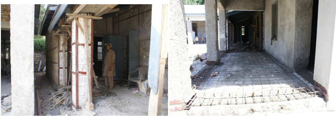
Figure 12. Strengthening of stone masonry columns (left) and adding tie beams and slab on grade (right)
