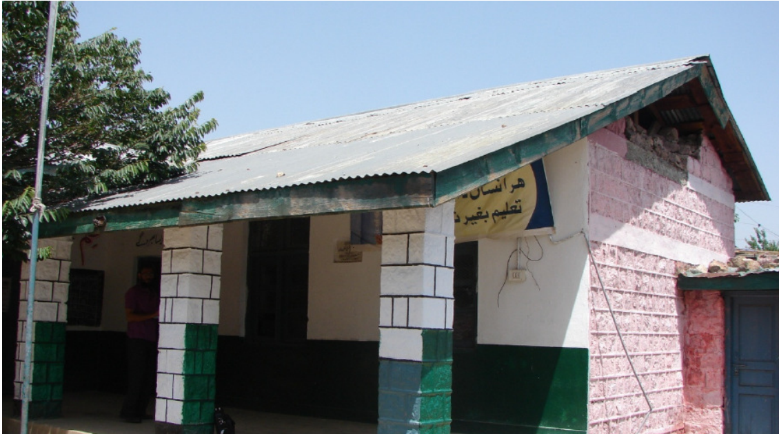
Figure 6. Out of plane failure of the gable wall in a school building
