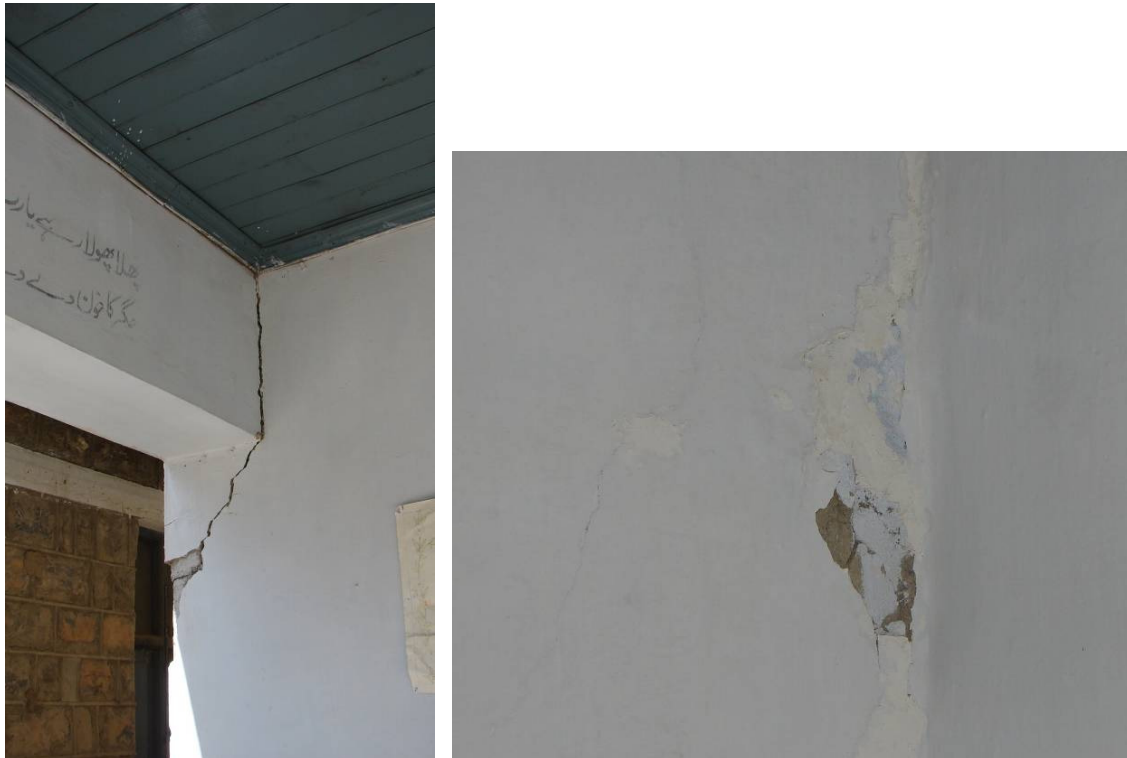
Figure 5. Typical cracks at openings (left) and wall junctions (right)
