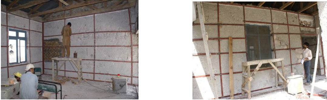
Figure 16. Placement of the vertical and horizontal steel straps – short wall (left) long wall (right).
