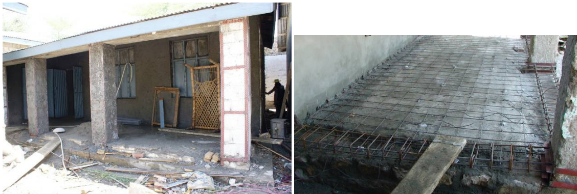
Figure 17. Retrofit of masonry columns (left); new slab on grad and plinth level tie beams (right)
